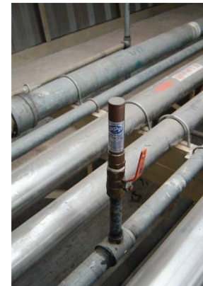
WATER HAMMER ARRESTER
